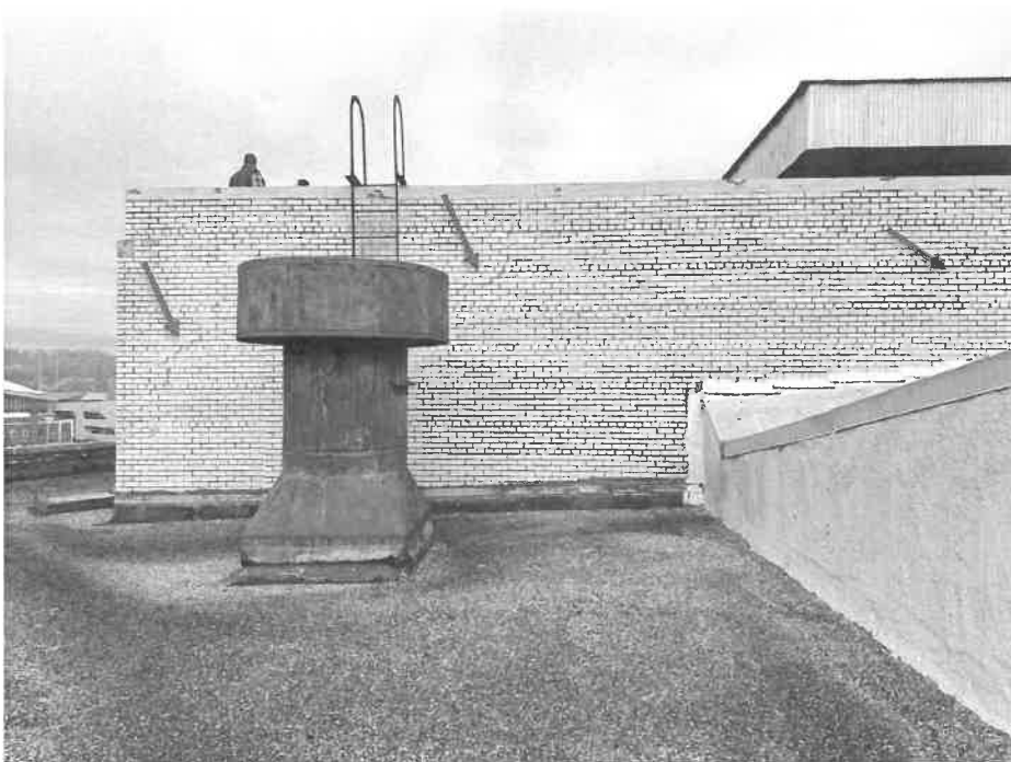
Photo 20: Step Cracking in Brick Masonry at Upper Penthouse
