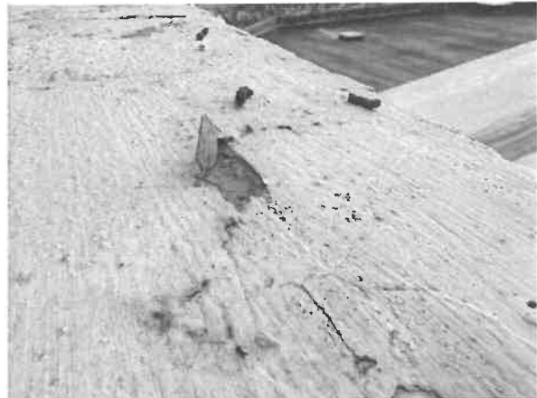
Photo 31: Typical Coating Failure at Parapet Coping Stone
