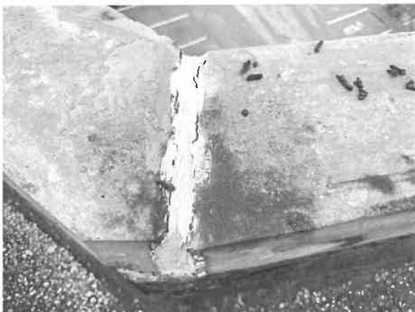
Photo 32: Sealant Joint Failures
