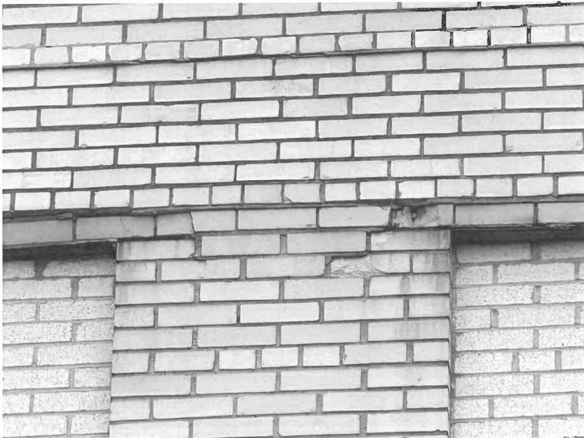
Photo 15: Displacement of Brick Masonry and Corrosion of Steel Lintels
