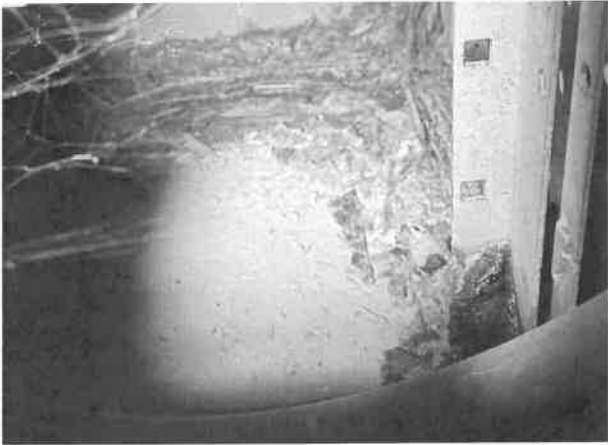
Photo 54: Interior of Switchboard - Rust Around Base of the Gear
