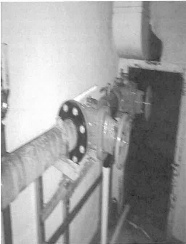
Photo 46: Main Water Service and Backflow Preventer
