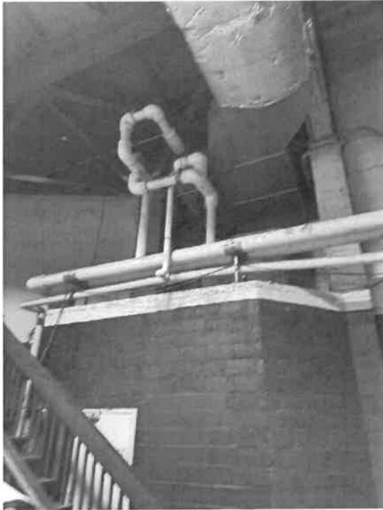
Photo 63: Stage Fan System
