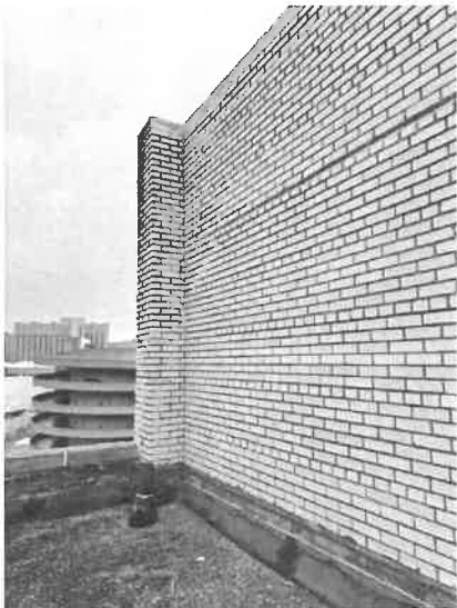
Photo 17: Displaced Brick at Parapets
