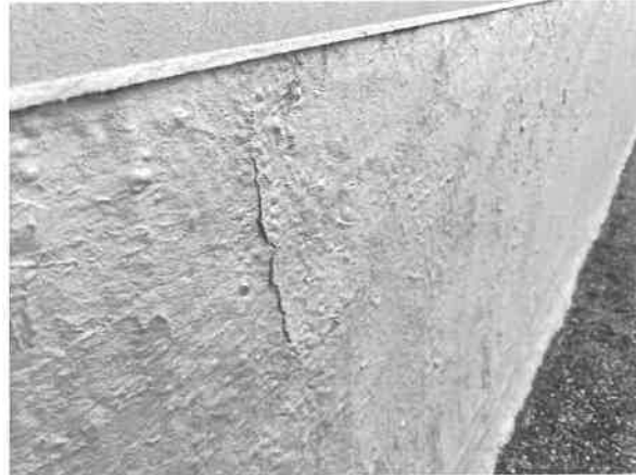
Photo: 35 Coating Failures at Sheet Metal Roof
