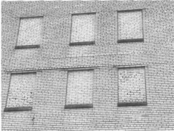
Photo 13: Displaced Brick at Faux Windows
