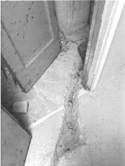
Photo 40: Trench Leading to Sump Pump
