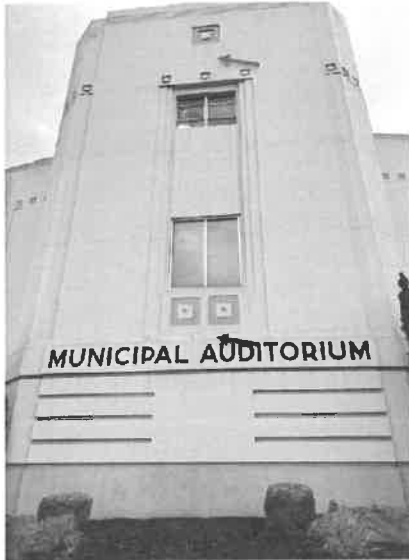
Photo 23: Vertical Cracking in Cast Concrete Façade
