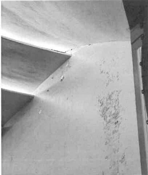
Photo 41: Typical Interior Plaster Damage in Auditorium
