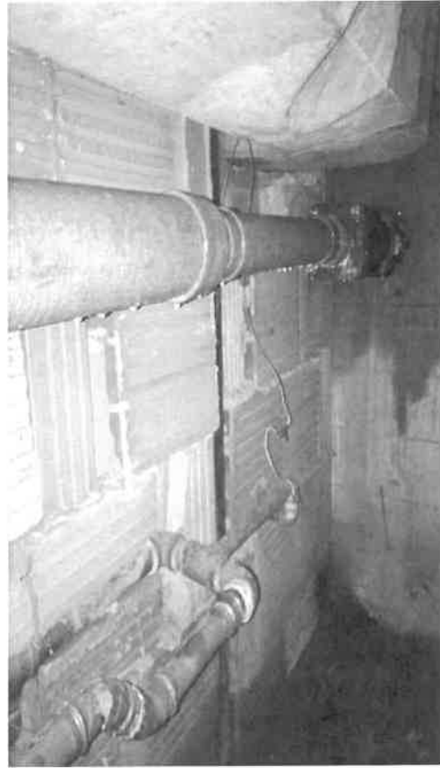
Photo 47: Copper and Galvanized Piping
