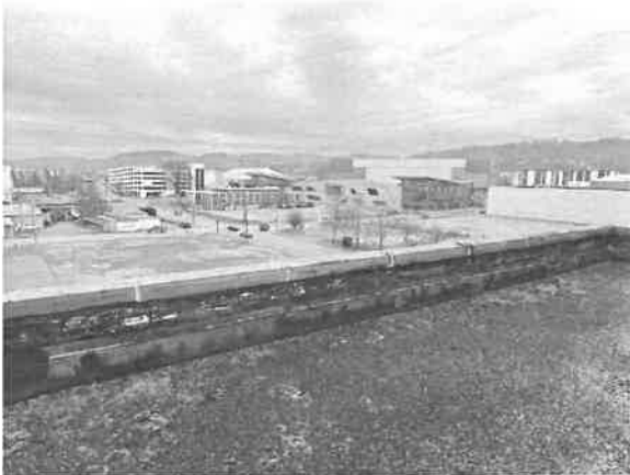
Photo 27: Typical Staining and Biological Growth at Roof Assembly
