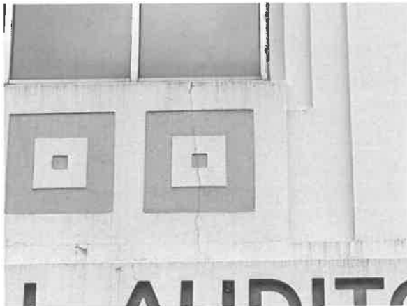
Photo 25: Vertical Cracking at Bottom of Wall
