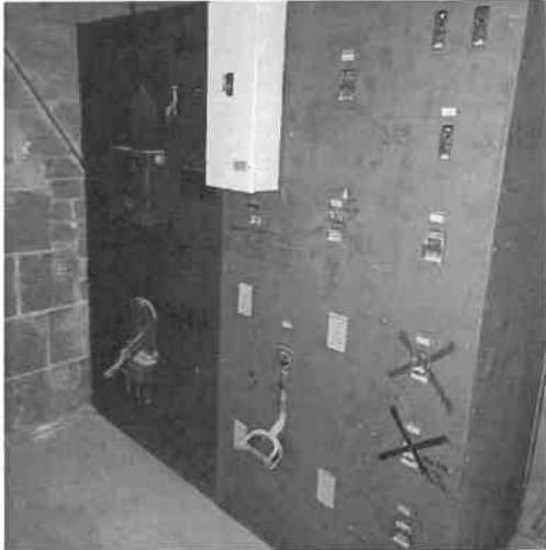
Photo 56: Dilapidated (Abandoned?) Gear in Penthouse
