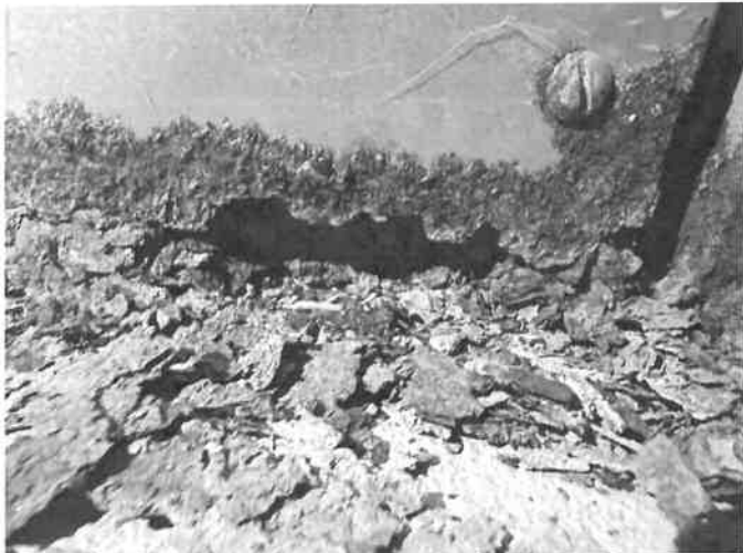
Photo 55: Exterior of Switchboard - Rust Around Base of The Gear
