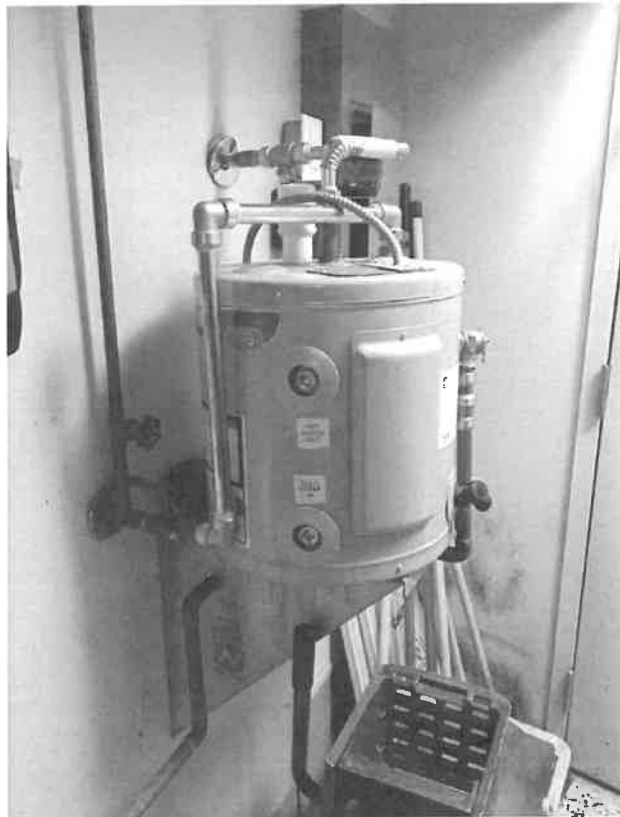
Photo 49: Electric Hot Water Tank
