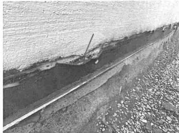
Photo 28: Pocket in Roof Termination
