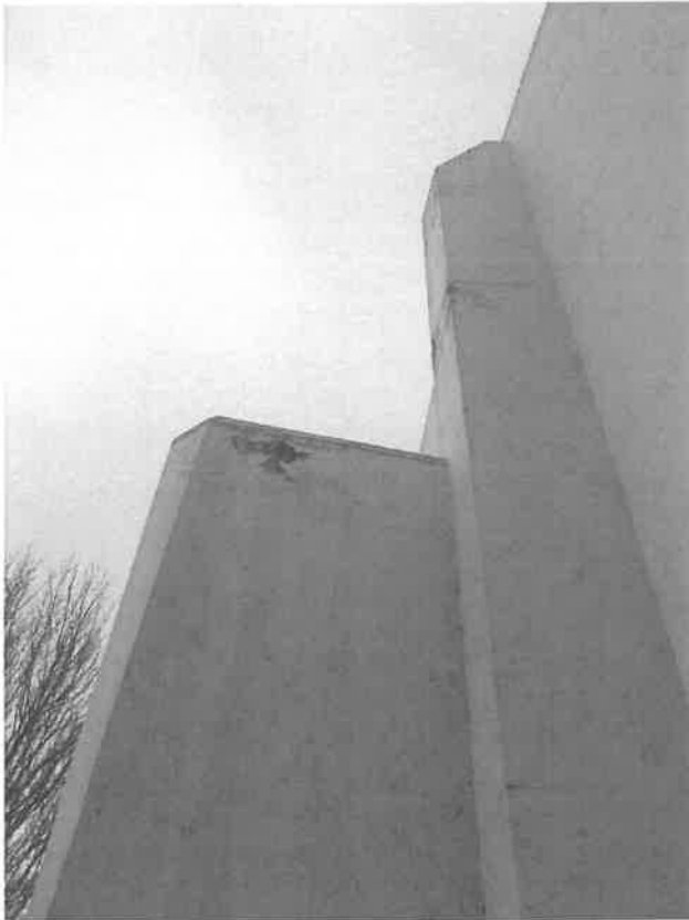
Photo 5: Evidence of Water Infiltration
