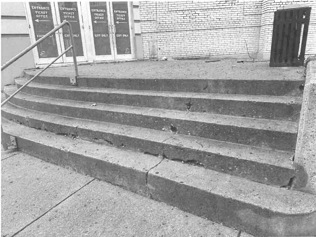
Photo 45: Cracking in Concrete Stairs
