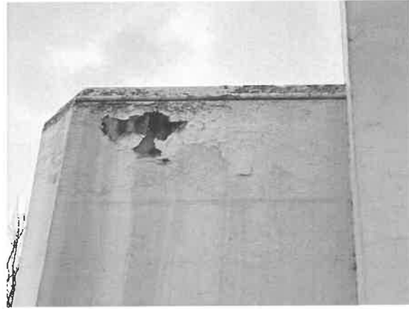
Photo 26: Paint Failures at Cast Concrete Façade
