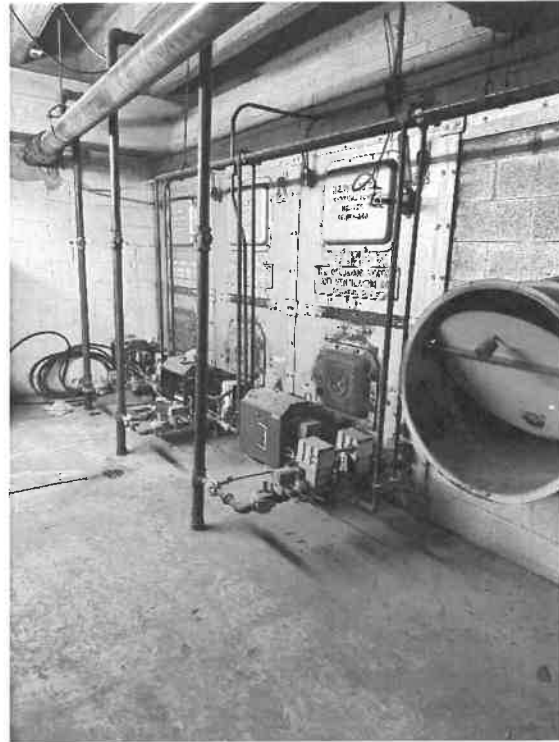
Photo 60: Existing Columbus Air Systems Unit
