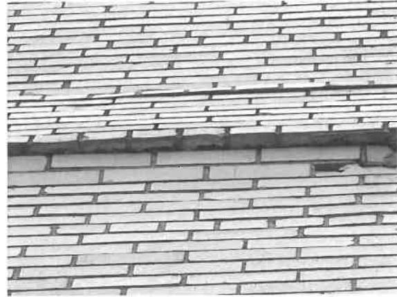
Photo 14: Displaced Brick at Faux Windows
