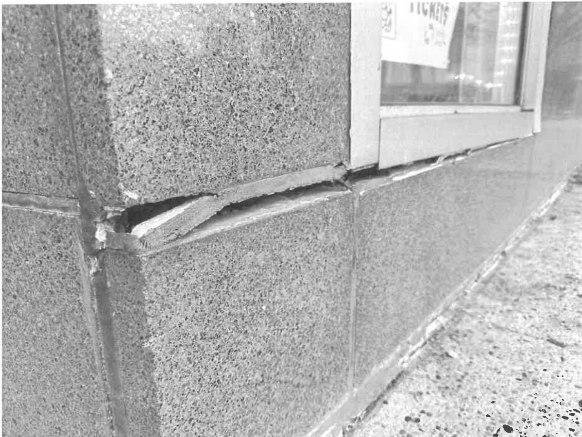
Photo 43: Separation in Joint in Granite Panels and Around Storefront Window
