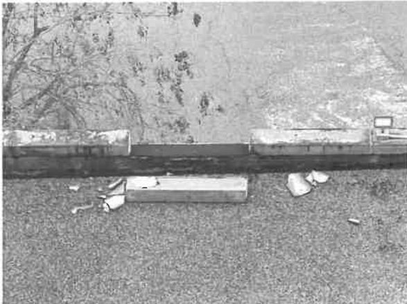
Photo 30: Displaced Coping Stone Unit
