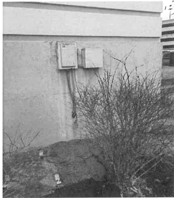
Photo 58: Abandoned, Unlocked with Exposed Wiring*
