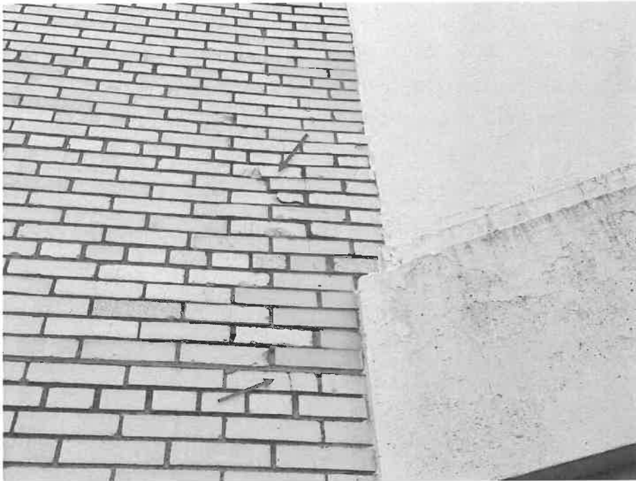
Photo 21: Cracking of Brick Masonry at Concrete Wall
