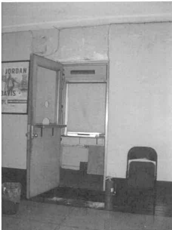
Photo 8: Interior Evidence of Moisture Infiltration
