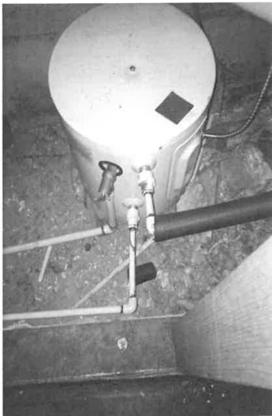
Photo 48: Electric Hot Water Tank
