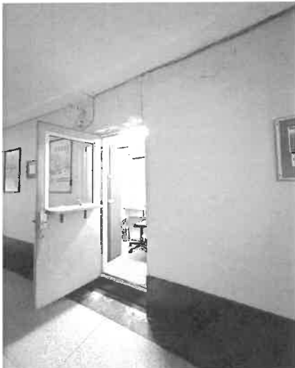
Photo 36: Interior Plaster Damage at Ticket Office
