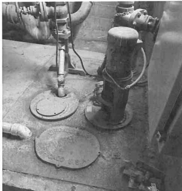
Photo 51: Duplex Sewage Ejector
