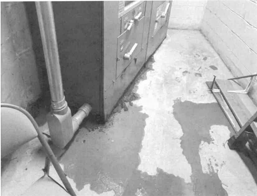
Photo 52: Water Seeping Out from Switchboard
