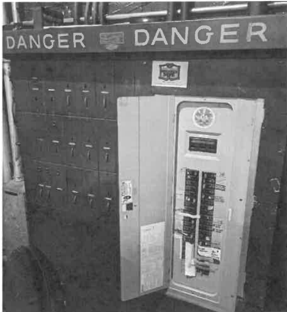
Photo 57: Abandoned Stage Dimmer - Retrofitted With Panelboard Compartment
