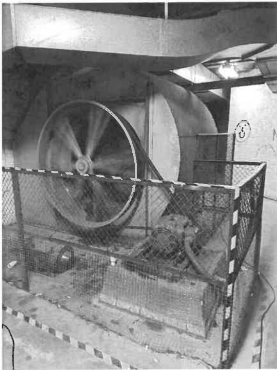
Photo 61: Large Blower Fan
